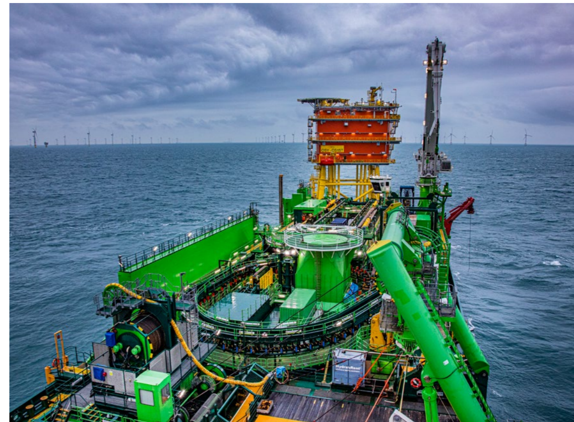
BELGIUM At the SeaMade wind farm, our cable installation and multipurpose vessel 'Living Stone' successfully completed the pull-in of two export cables into Elia's Offshore Switch Yard
